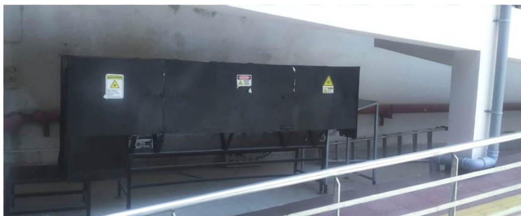
Installation at main gate, IIT Jammu
